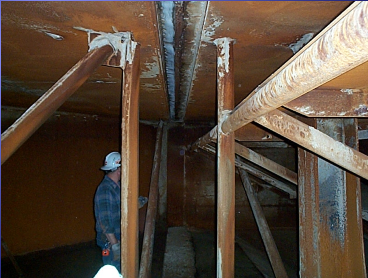
Pleasant Prairie Power Plant – 9'6" high x 38'0" wide duct
